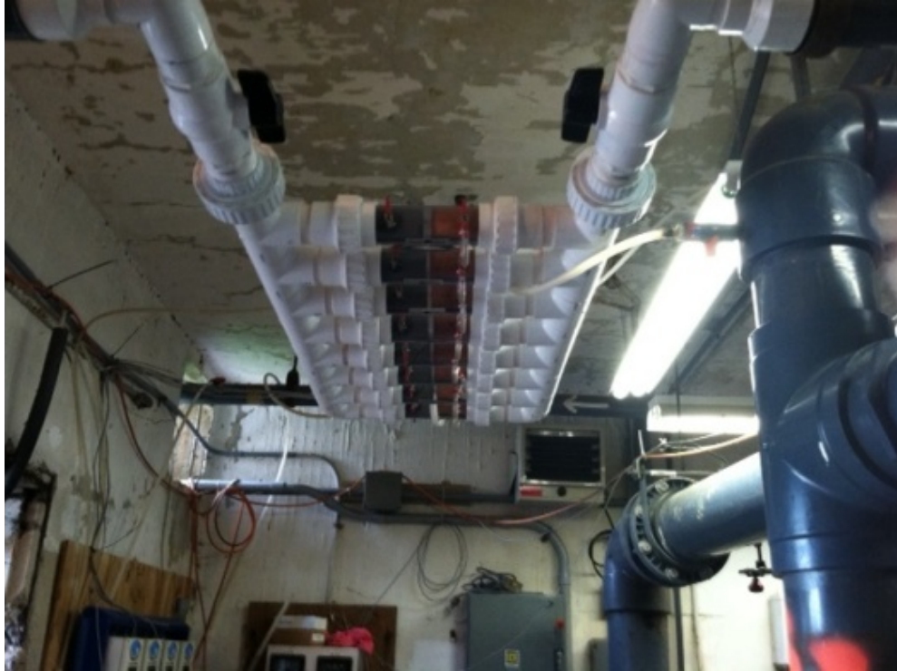
4 ECOsmarte Controllers & 8 Cu/Oxy 2" Anode Chambers
